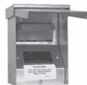
U3800 with GFCI Receptacle
